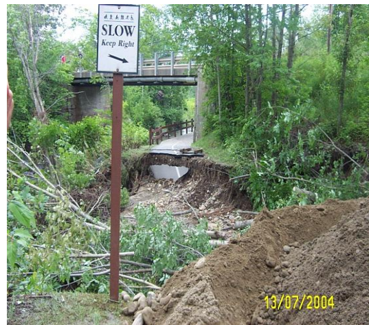
In 2004, a section of the Stowe Recreation Path upstream from the Luce Hill Rd. Bridge was replaced after a heavy rainstorm eroded the bank of the West Branch River.
