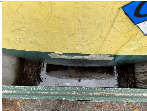
Photo 15: Inside of secondary containment for two 350-gallon gasoline and diesel fuel ASTs
