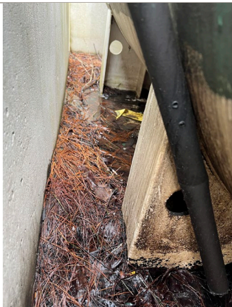
Photo 11: 350-gallon AST secondary containment
