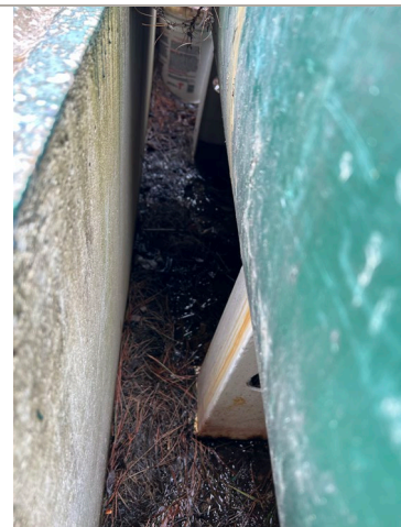
Photo 16: Inside of secondary containment for two 350-gallon gasoline and diesel fuel ASTs
