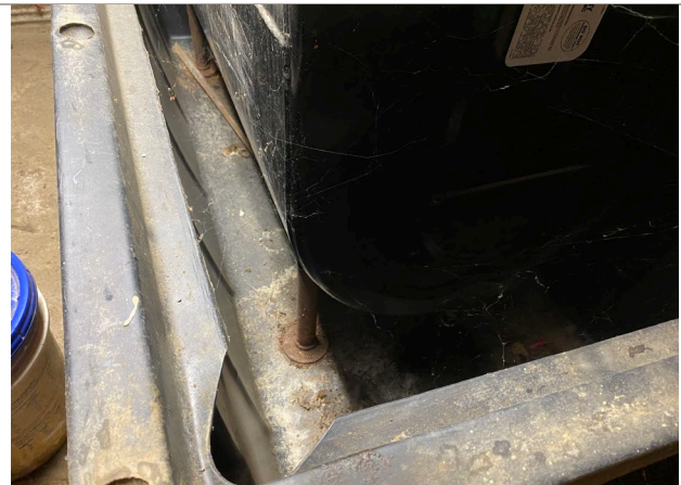
Photo 12: 275-gallon AST secondary containment
