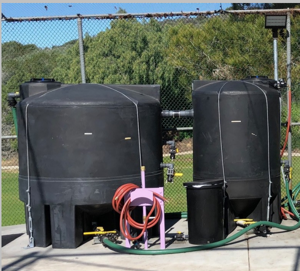
CLARIFIER & WATER STORAGE
