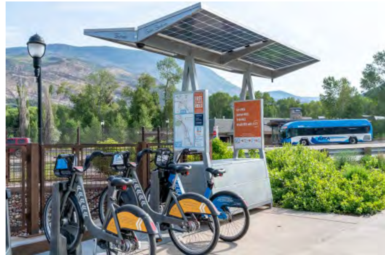
Example of Solar E-Bike Charging Station in Colorado
