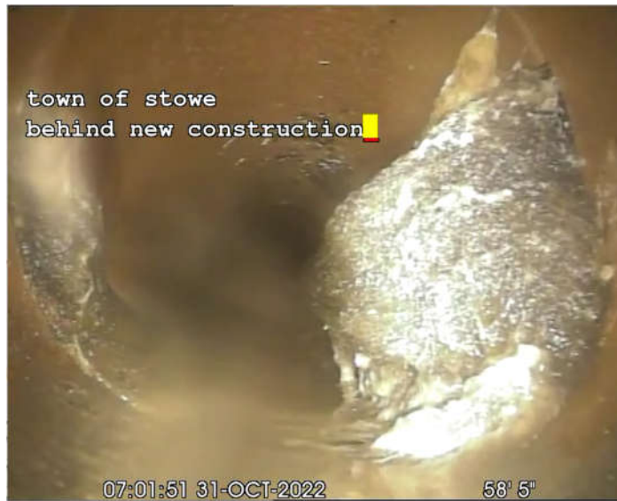
58 ft: Roots entering pipe between pipe segments, typical of 6 locations
