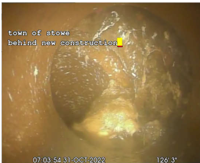
126 ft: Major offset with exposed soil, camera could not pass this location (aprx. 5/6 of pipe inspected)
