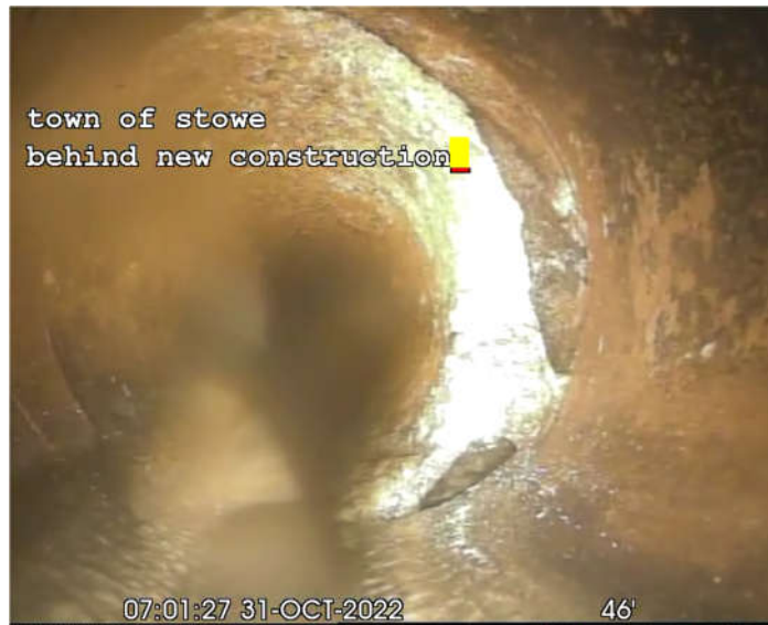
46 ft: offset pipe with exposed soil
