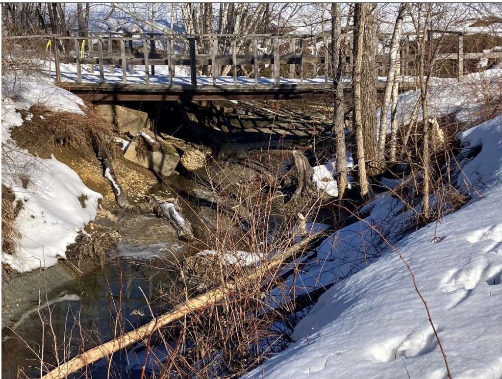
VIEW EAST WITH NORTH ABUTMENT BLOCK COLLAPSE INTO STREAM
