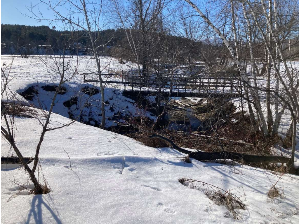
VIEW WEST WITH FLANKING SCOUR AT SOUTH ABUTEMENT
