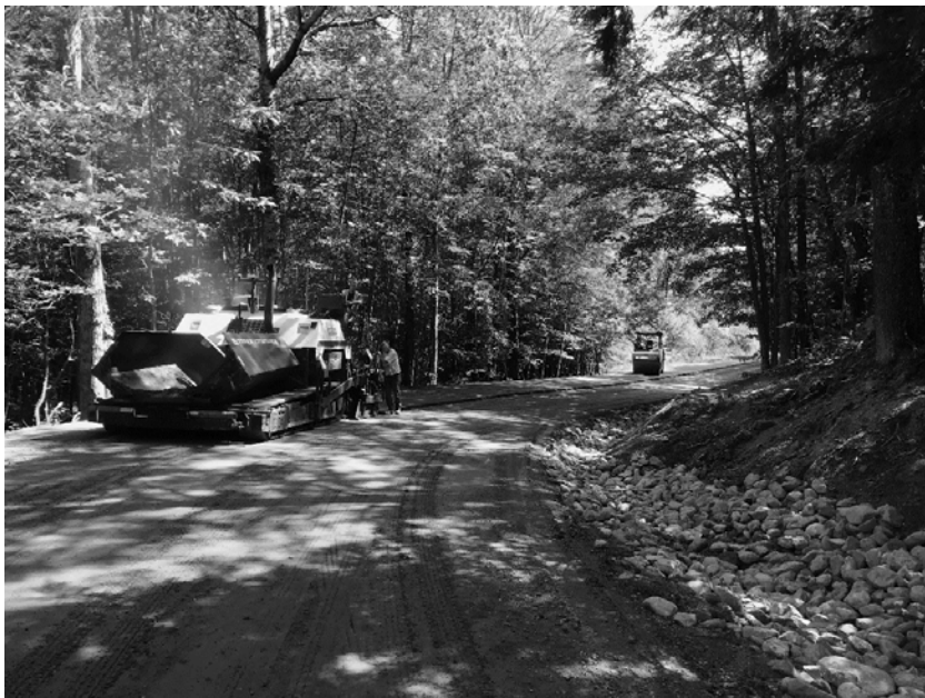
West Hill Road paving following drainage system improvements to meet Stormwater requirements.
