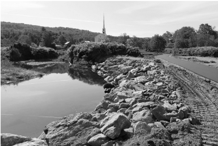
Streambank stabilization efforts completed along the Rec Path summer 2019, including a newly paved Rec Path up to Bridge 2.
