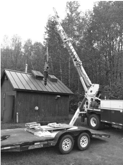
Stowe Water Department with the help of Stowe Electric airlifting a new pump through a roof access hatch at a Mountain Road pump station.
